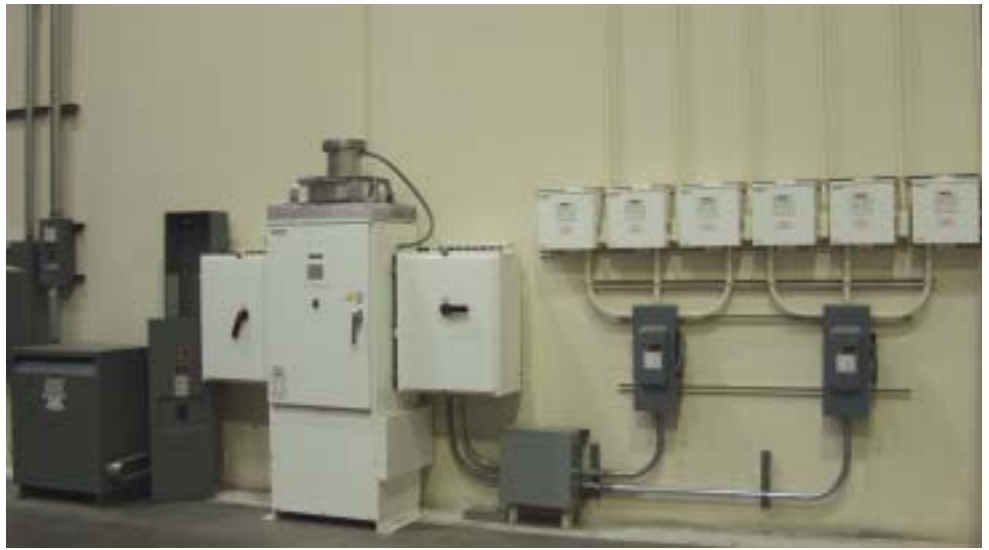
Final connections of all rooftop electric wiring to inverters and then to the utility grid.
