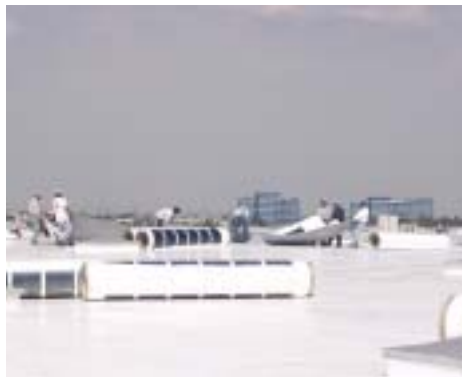
Workers from Southern California Roofing are installing the SR-2001 photovoltaic panels to the Sarnafil EnergySmart Roof membrane.
