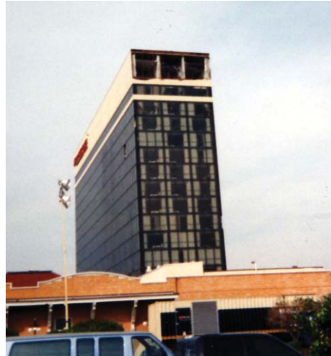
Crowne Plaza Grand Hotel, Pensacola, with the upper floors' walls blown in.
